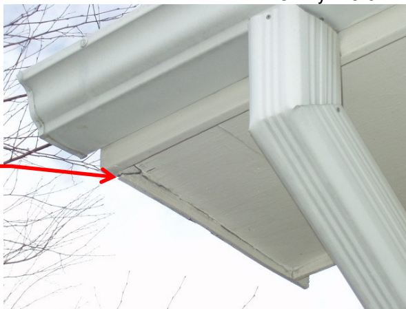
Figure 2: Fascia Board on N.E. Corner of Front Parch
